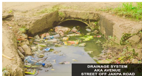
Fig 1.2: Refuse in Aka Avenue Drainage
