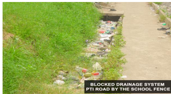
Fig 1.1: Refuse in PTI Road Drainage
